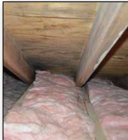
➤ Attic-insulation baffles could have been used here to prevent the insulation from blocking the intake vents. Photo courtesy of Sam Rosario, Liberty Construction Inc., Worcester, Mass.
